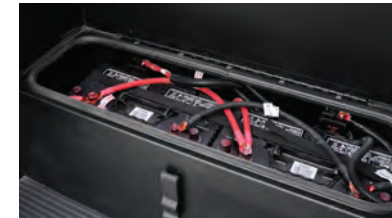
Two batteries in a single housing for easy access. (One battery LE and Transit)
